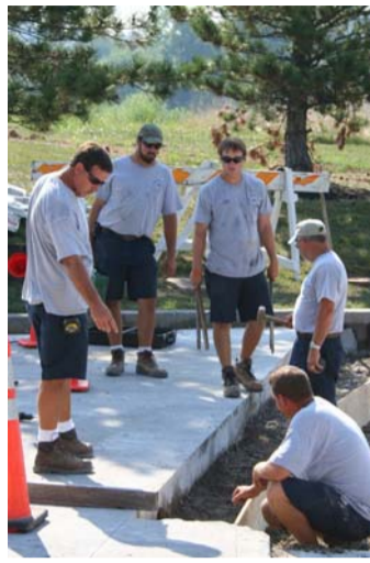
Dave Becker (left) directs his crew as they prepare Meridian Drive for repaving.
